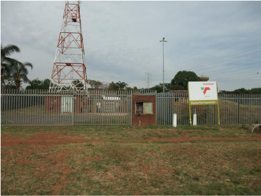
Figure 13: The Elardus Park depot. Also note the white markers indicating the position of the pipeline.
