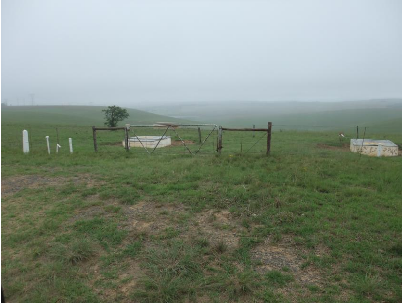
Figure 48: Note servitude for the pipeline and inspection chambers in a landscaped environment.
