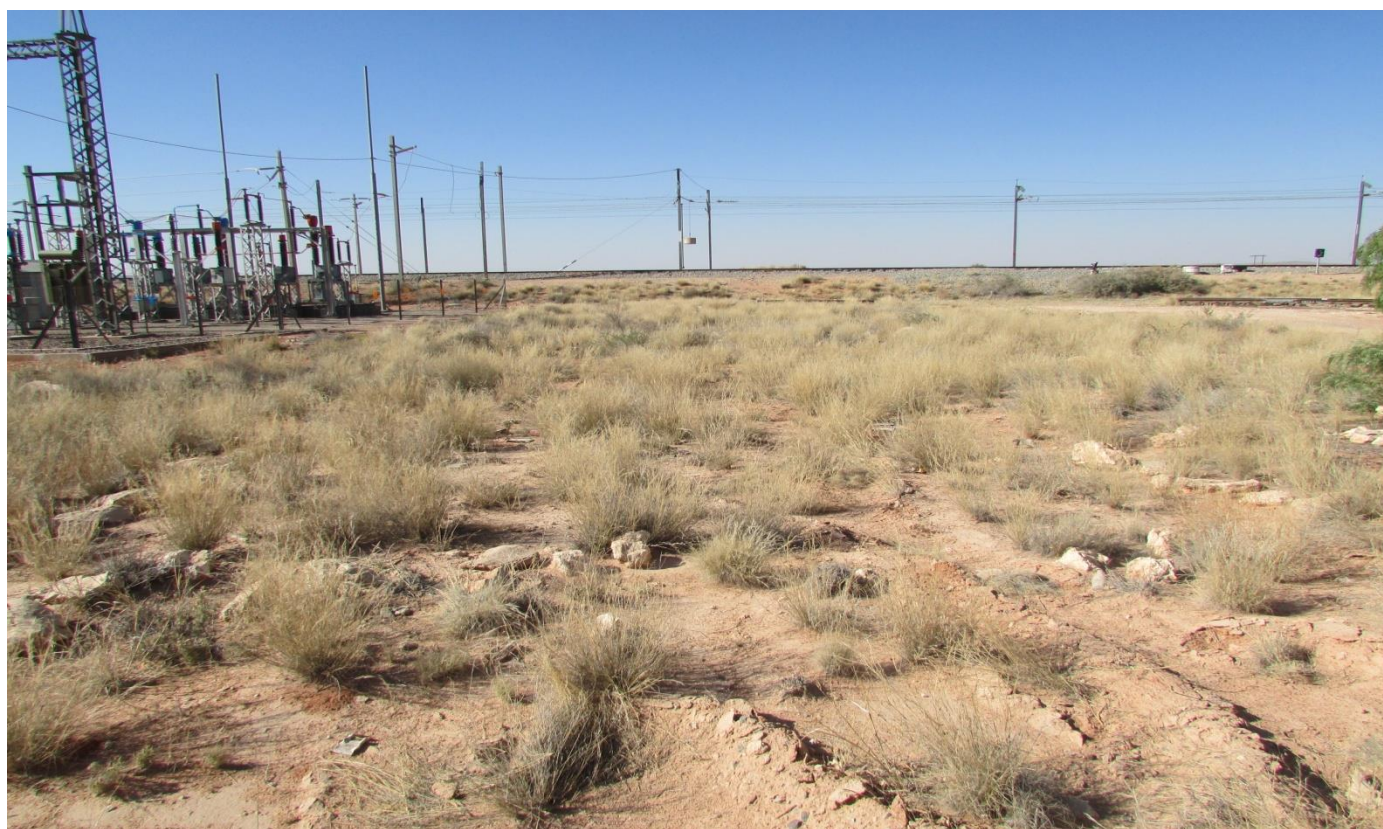
Figure 4: An over view of Garona substation and Transnet Railway Line in the background.
