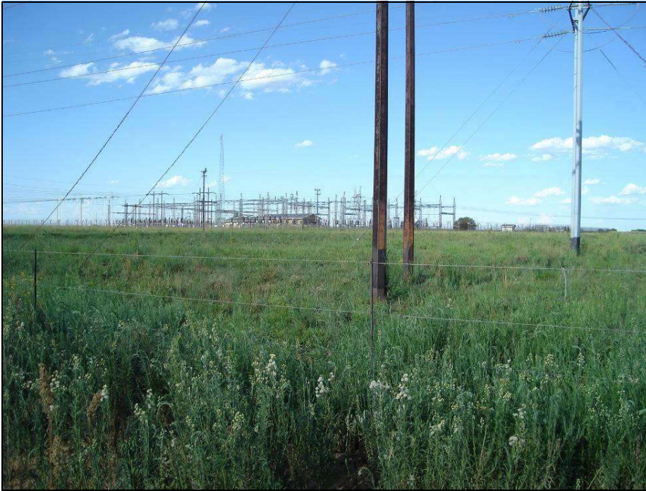
Fig.22 Point 22. Mercury Sub-Station between Orkney and Viljoenskroon.
