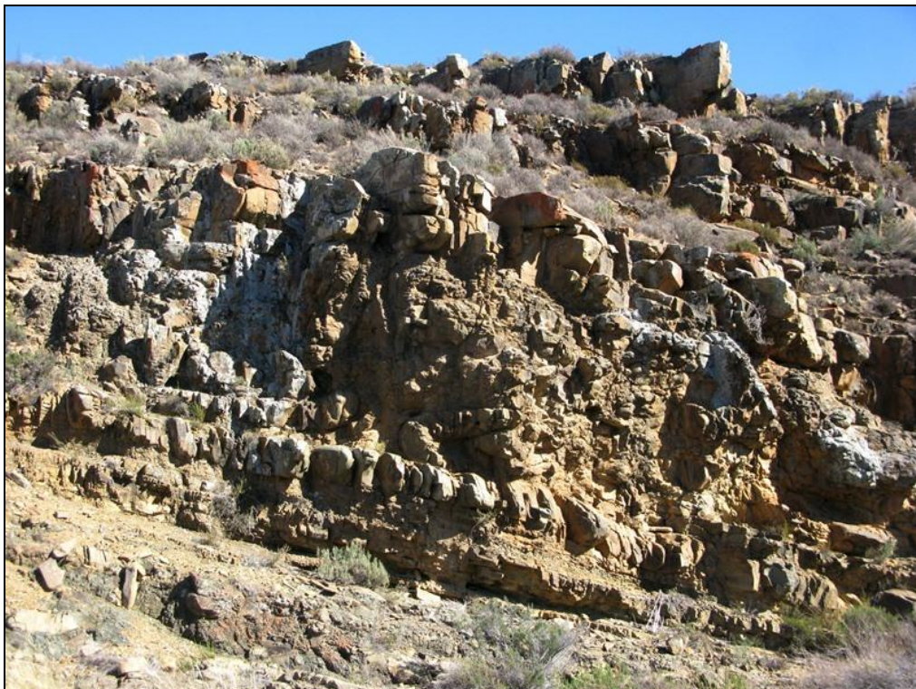
Figure 13. Riverine cliff exposure of a thick package of wackes of the Waterford Formation, locally showing high levels of soft-sediment deformation and disrupted bedding, Barendskloof, Barendskraal 76 (Loc. 213).
