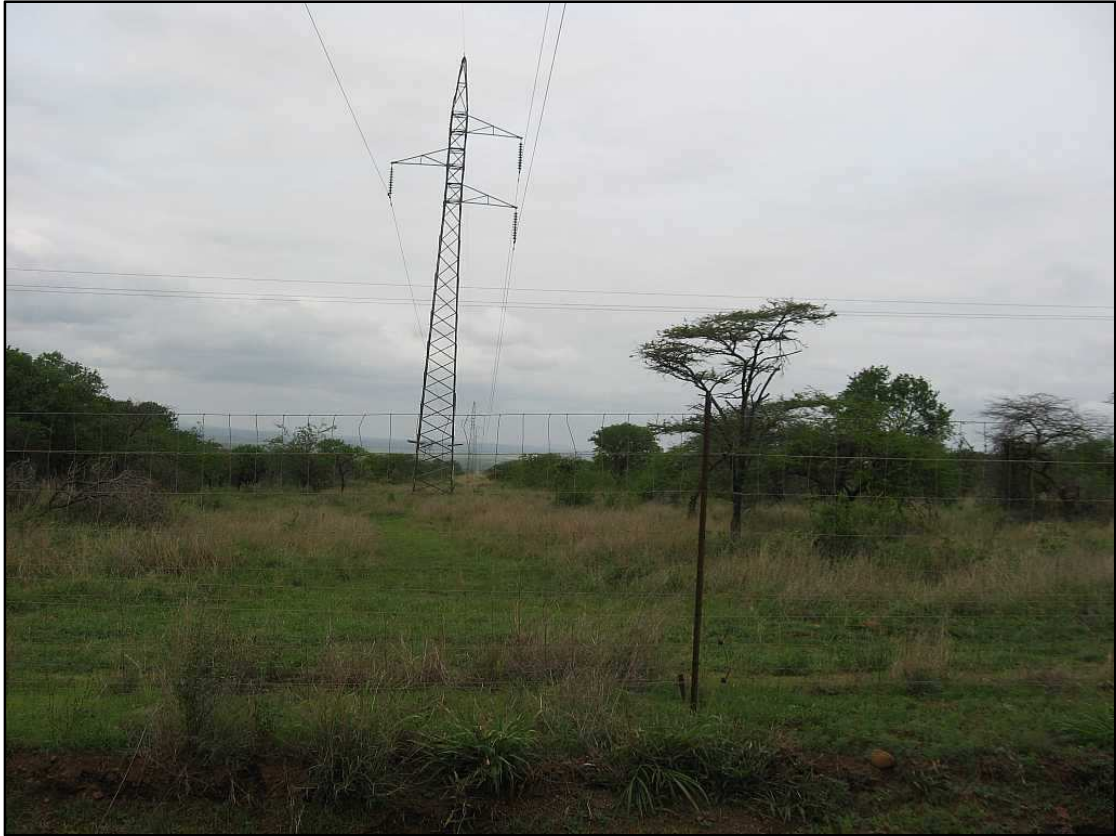
Figure 14 – Existing 132kV line
