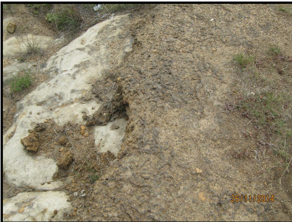
There is some concern with the property (portion 19) on which the Department of Agriculture wants to construct an abattoir. The area has a small inlier of shale present, if the footprint of the building can be moved due to the large extent of the site and foundations are not deeper than 600mm it may be possible to avoid building on the shale. If the shale covers the entire site then the topsoil, subsoil and overburden must be surveyed for fossils and Mitigation is needed for the shale layer.
