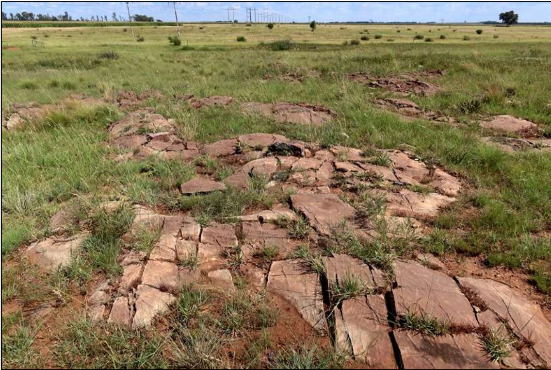
Figure 9: Extensive exposure of well-jointed, pale brown Malmani carbonate bedrocks to the south of the proposed on-site substation, just north of the existing power line. Note the pronounced undulating surface with low ridges and swells that is possibly related to large stromatolitic domes.
