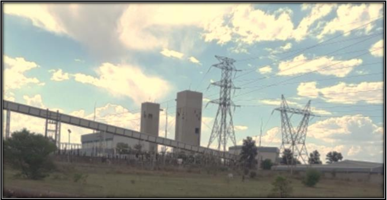
Figure 9: Existing Vaal Reefs Ten Substation.
