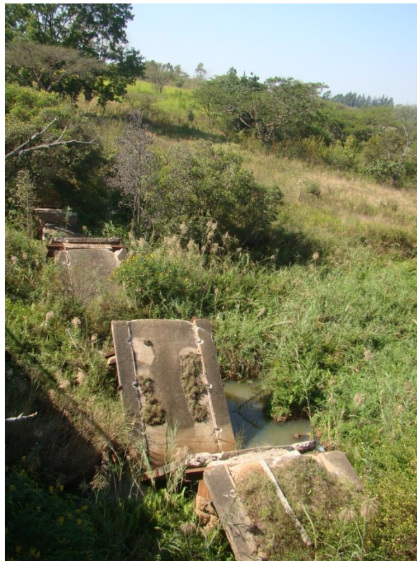
Fig. 10: The original bridge across the White River was damaged on purpose to prevent people from using it.
