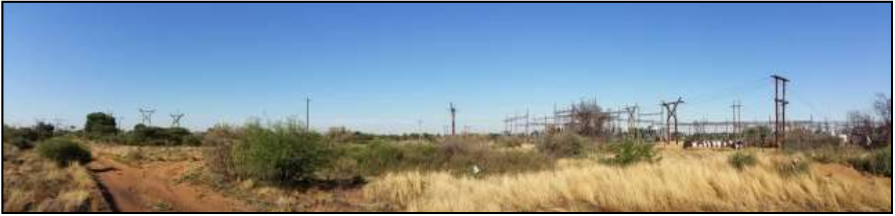
Figure 11: The substation of Hotazel on the western edge of the town.
