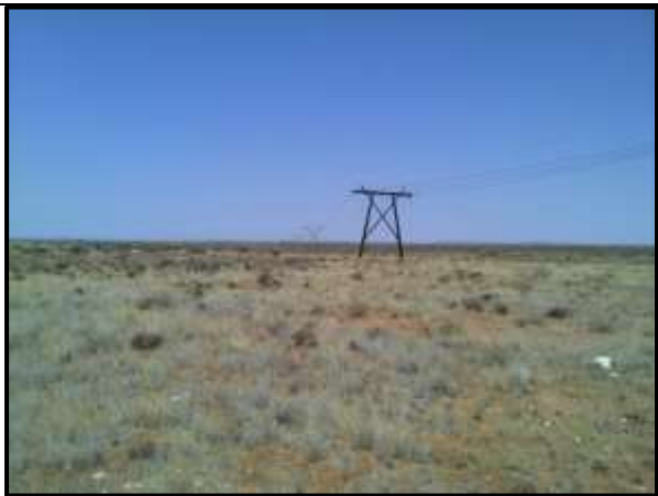
Figure 9: Existing powerlines in the eastern section.
