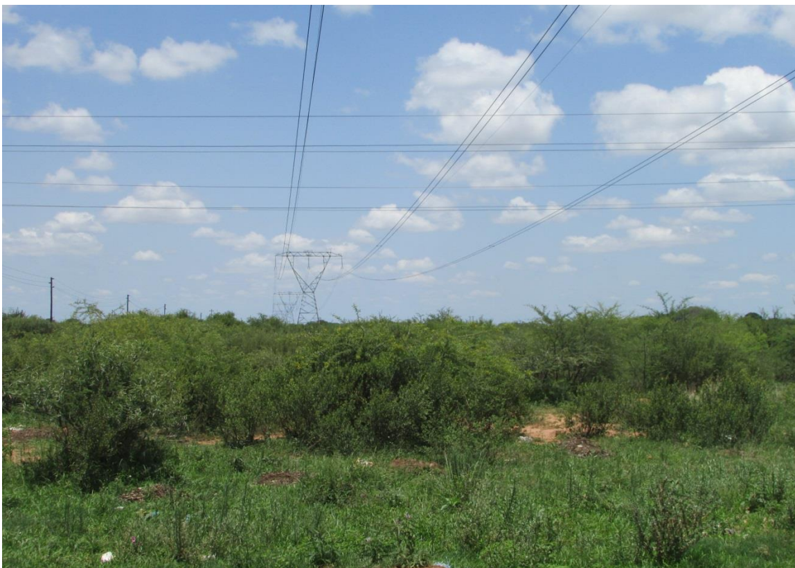
Figure 20: A view of a section of the Grid Connection Corridor running from the substation south towards the Phala SPP study area.
