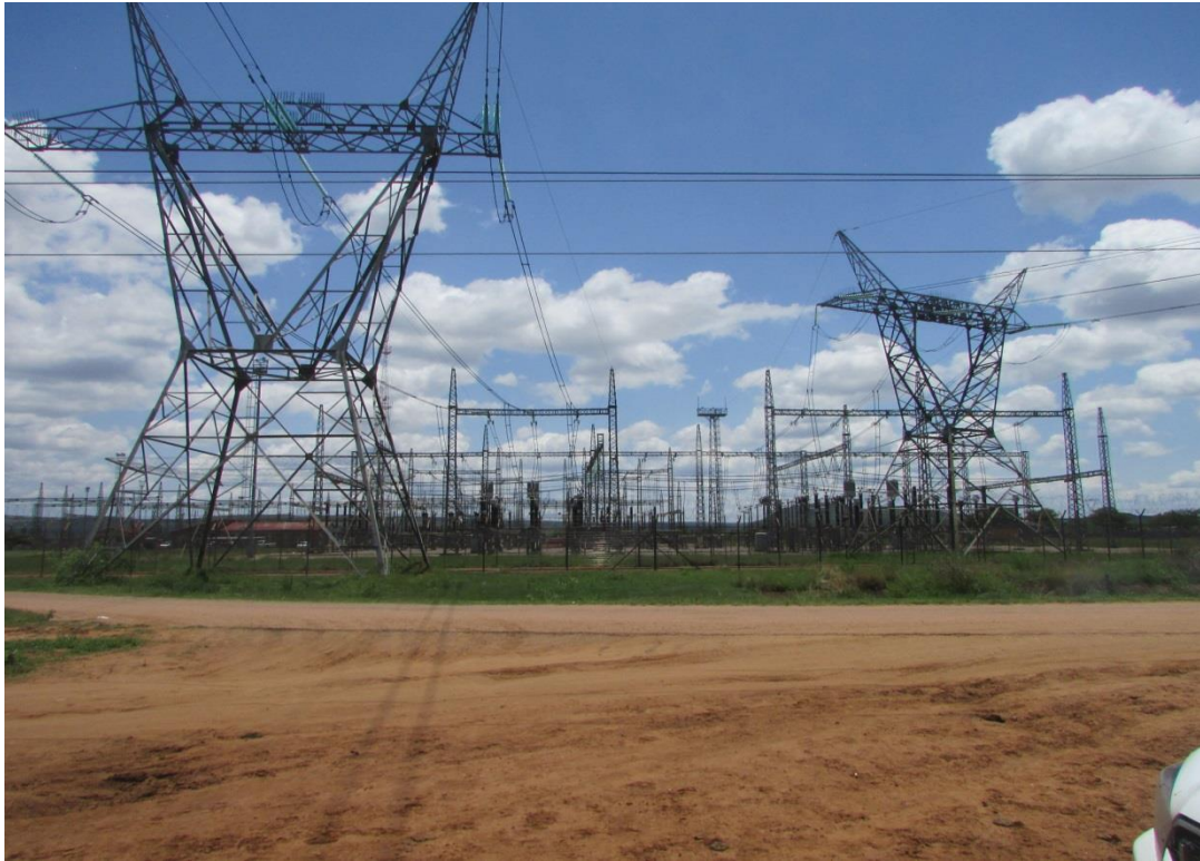
Figure 19: The Warmbaths Substation where the Phala SPP will connect using the existing Eskom lines.
