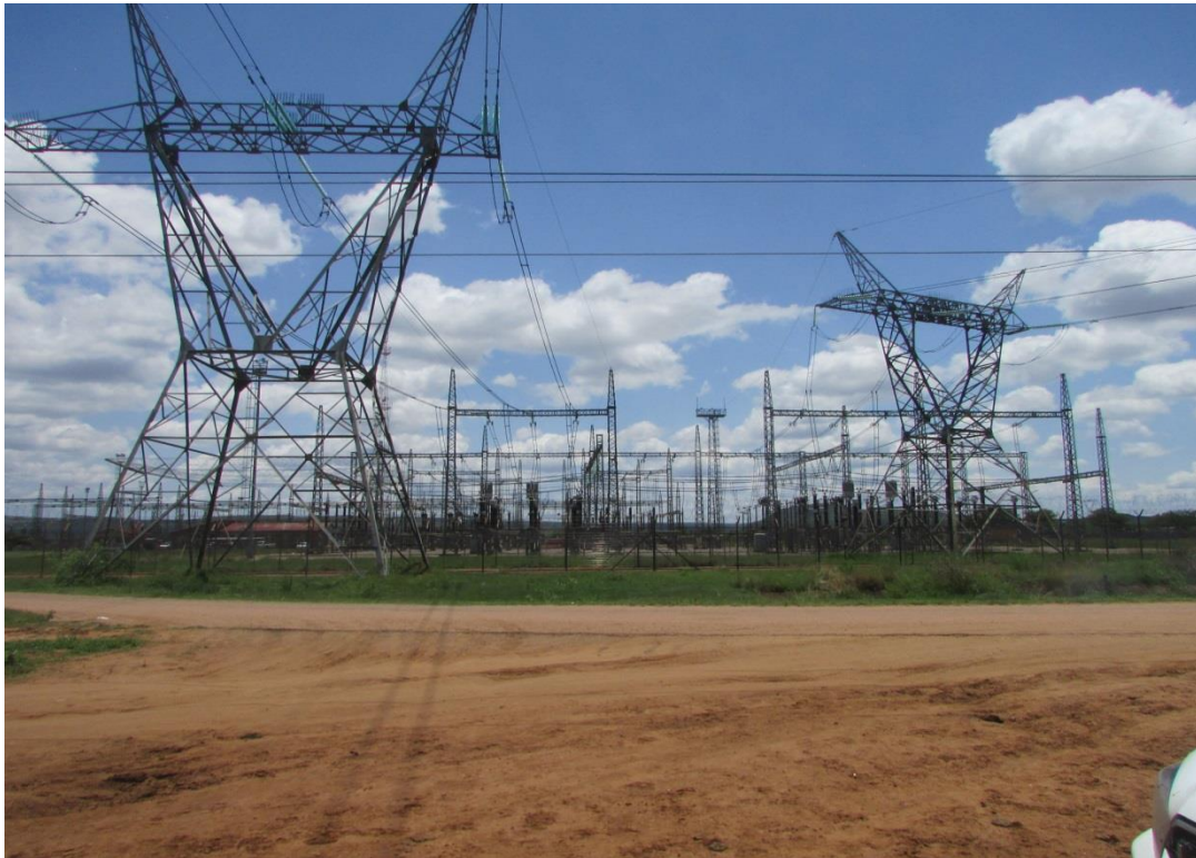
Figure 19: The Warmbaths Substation where the Phala SPP will connect using the existing Eskom lines.
