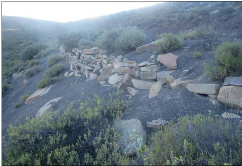
Figure 19: View towards the south of a section of the drystone walling supporting the road above the Riet River (waypoint 560).
