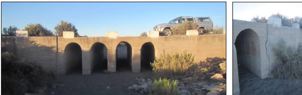
Figures 16 & 17: View of the largest built structure along the road (waypoint 561). It has been built of modern concrete and is showing signs of deterioration.
