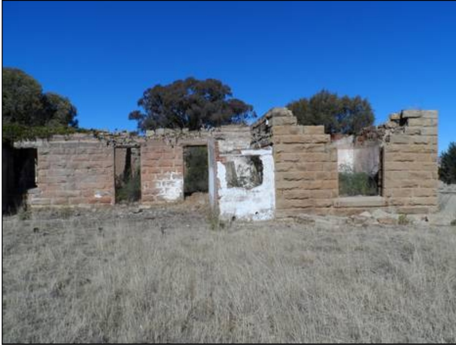
Figure 18 - South facade of the farmstead main farm house ruins. Note the red brick additions. Also note the white paint that dresses some of the sandstone bricks as well as the brick addition and the inside.
