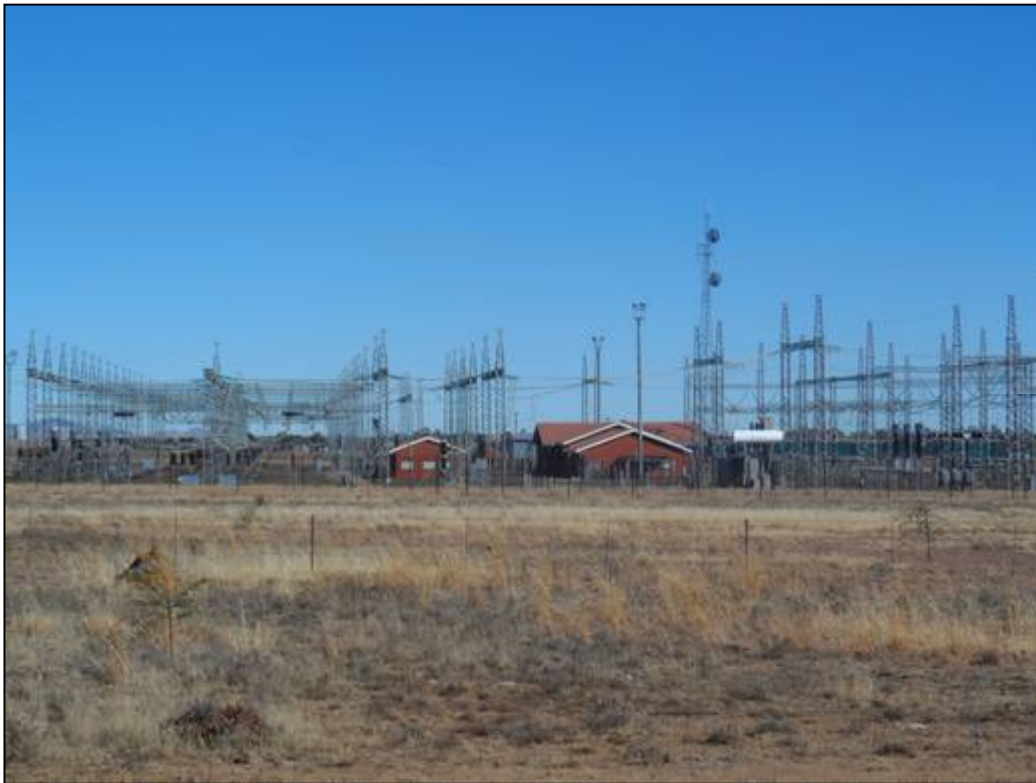
Figure 4 - Picture of the existing Substation.
