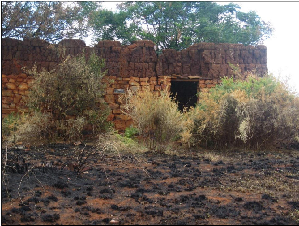
Figure 56 – View of utility building at WTR006
