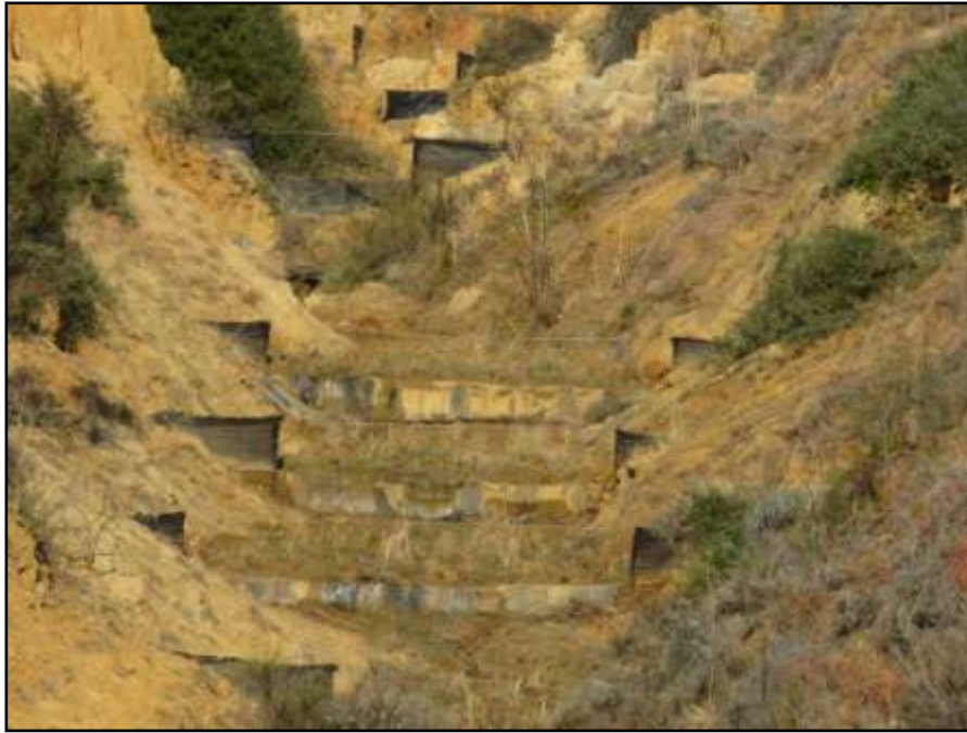
Fig. 3. Another example of soft intervention is a silt fence which reduces and stops erosion in dongas with small catchment areas by means of cheap and easily constructed structure. This is a photo shortly after construction.
