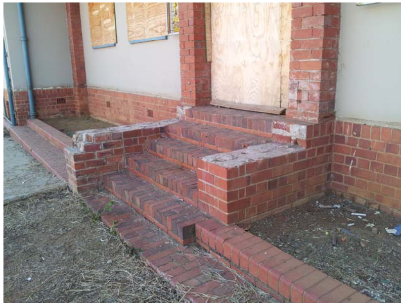
Figure 11: Damage to entrance on southern facade
