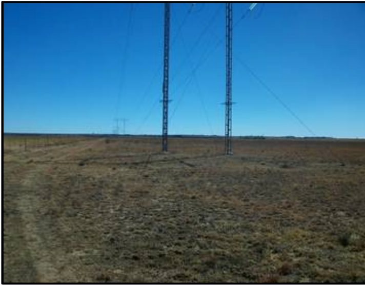
Figure 4. View of the power line forming the western boundary of the study area.
