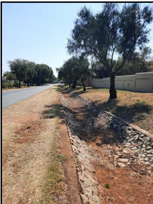
Figure 3.3. General site conditions - Drainage systems built onto the road reserves may be older than 60 years.
