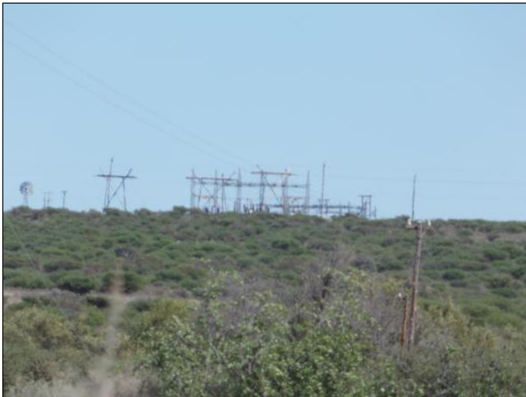
Figure 3. General Landscape and local sub-station
