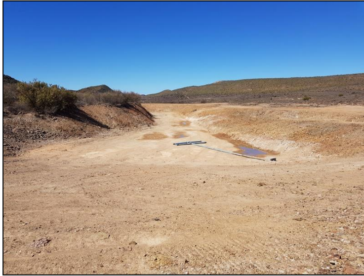
Figure 3-3: View of general surroundings at the site of the newly constructed dam subject to the S24G rectification.
