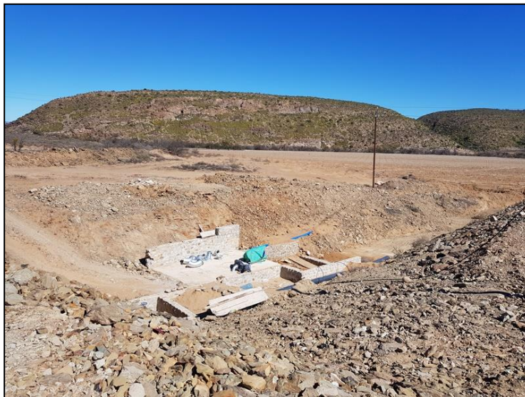
Figure 3-5: View of general surroundings at the site of the newly constructed dam subject to the S24G rectification.
