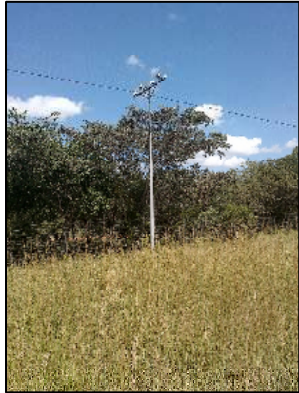
Figure 7-8. Overgrown vegetation and power lines running next to the road.
