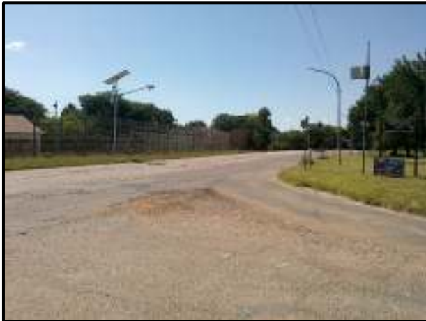
Figure 7-1. General site conditions- Road conditions near the extent of the Modimolle section of the upgrade.
