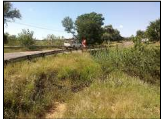
Figure 7-2. Klein Nyl River Bridge which will be replaced with a new, larger bridge.
