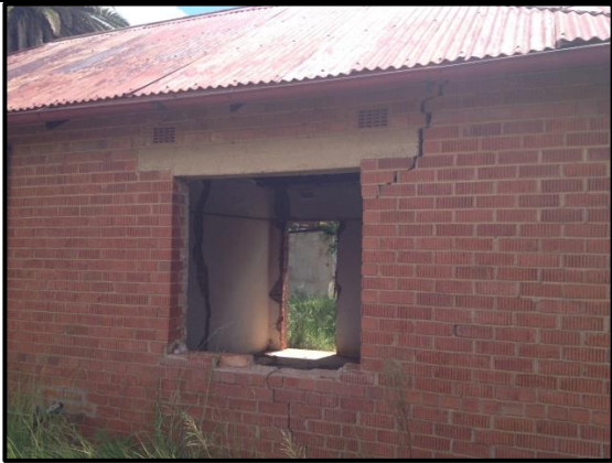
Figure 14: Windows and electrical connections have been looted from the structures.
