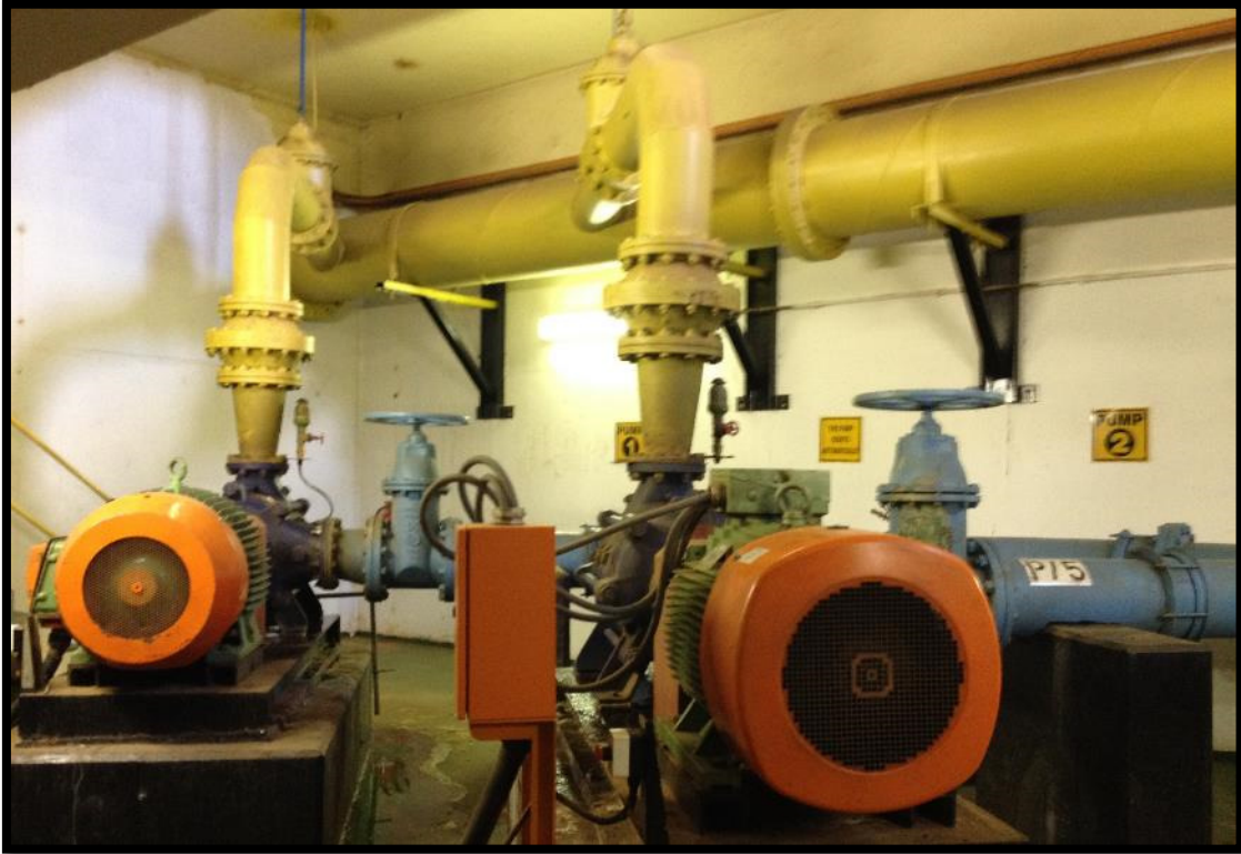
Figure 17: Existing pumps and motors at the Hospital Hill pump station, viewed from the side
