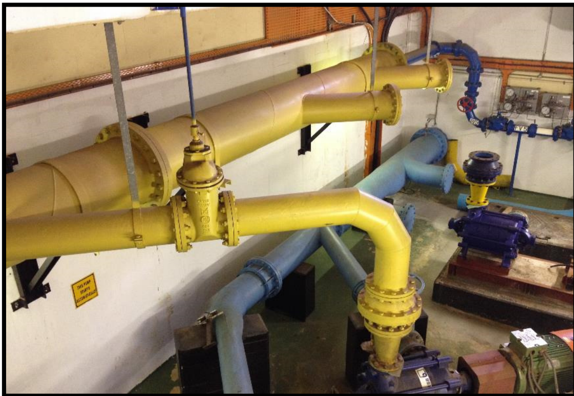
Figure 16: Inlet (blue) and outlet (yellow) pipes inside the Hospital Hill pump station
