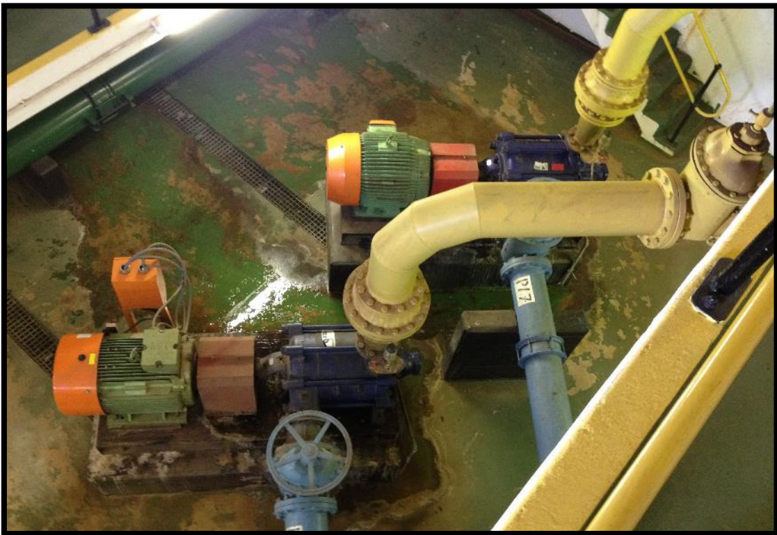
Figure 18: Existing pumps and motors at the Hospital Hill pump station, viewed from the top
