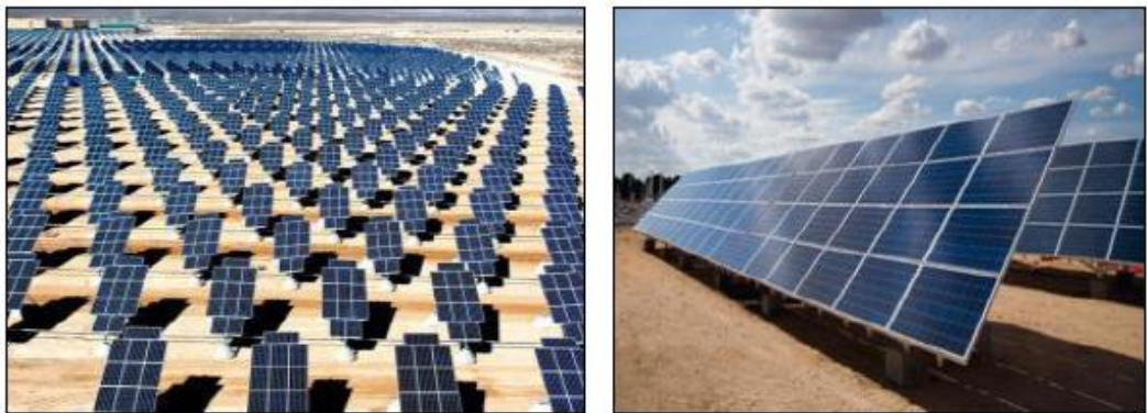
Figure 2. Example of a Solar PV installation (supplied by Digby Wells).
