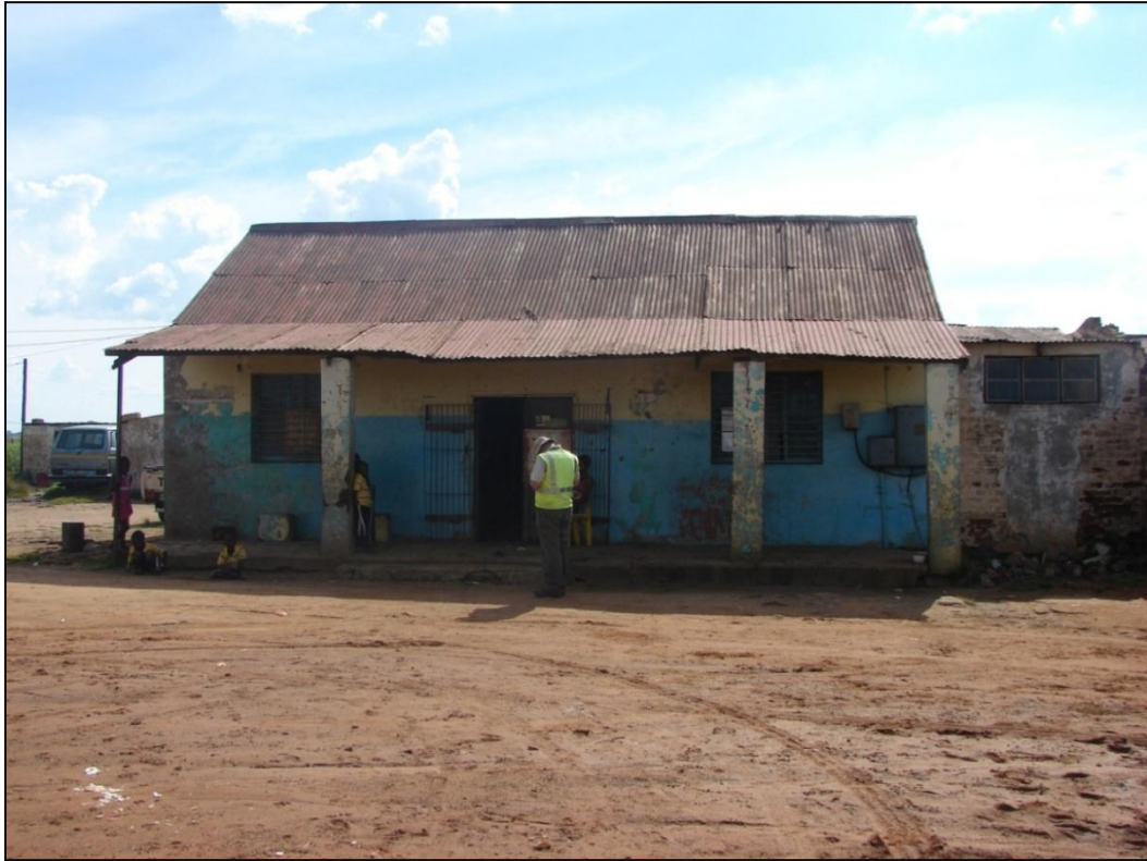
Figure 48 - Extension of the right end of the shop-view from front façade. © Tomose @ PGS.
