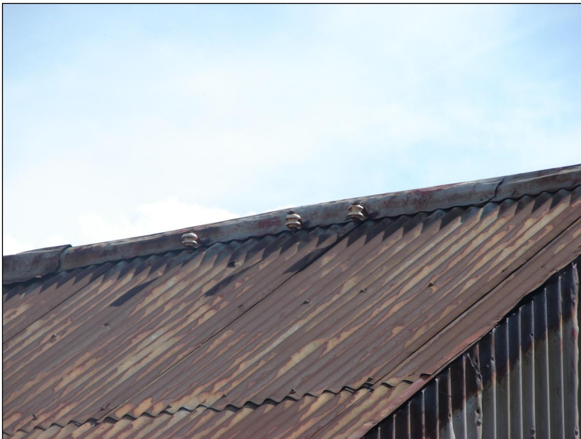
Figure 50 - Historic electricity port connections on the shop roof. © Tomose @ PGS.
