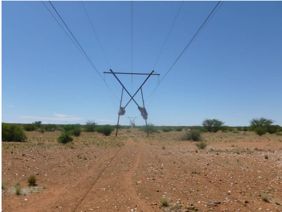
Figure 7: 132kv line looking west
