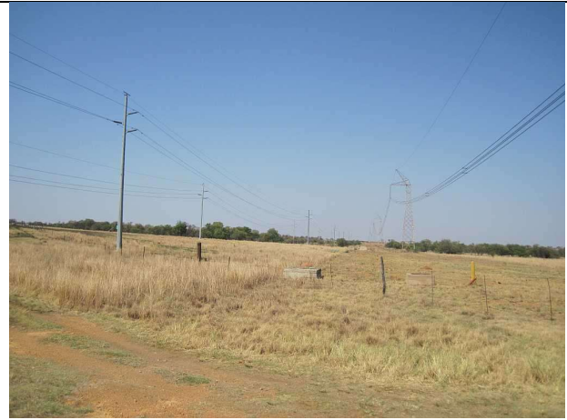
Figure 6. Cahora Bassa Powerline
