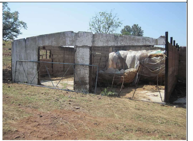
Figure 29. Cement brick ruin
