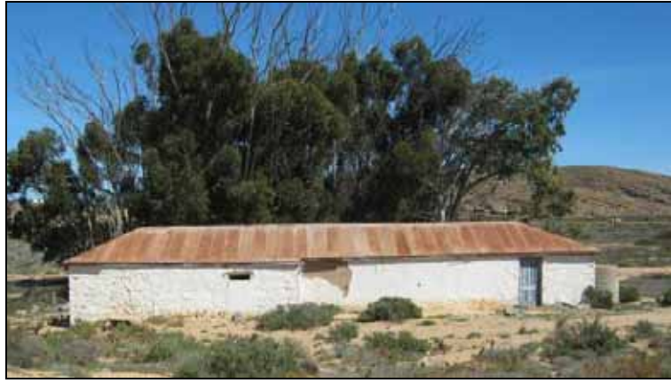
Figure 35: Derelict historical building at Grootmis.
