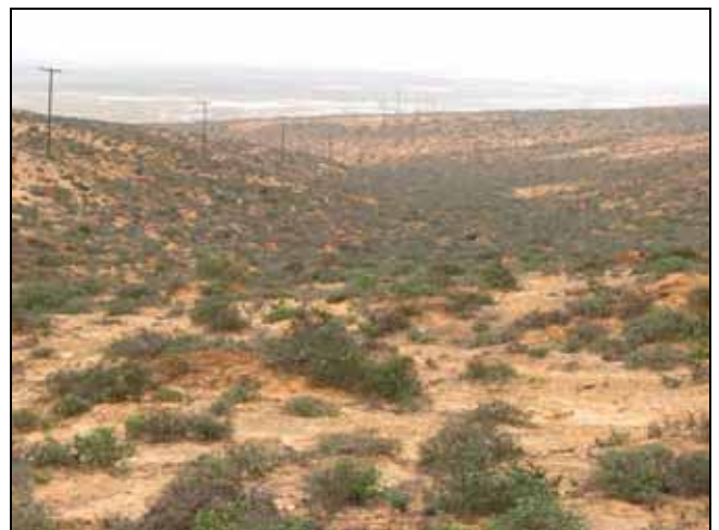
Figure 12: Power line crossing the southern part of the study area towards Kleinzee.
