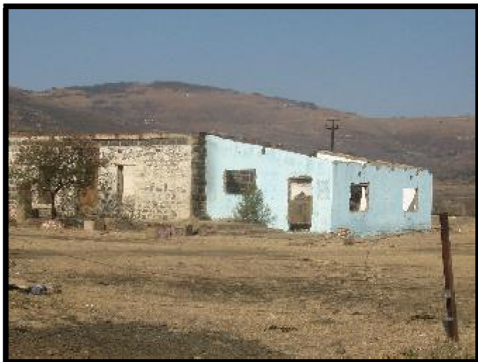
Figure 13. Trading Store 2. This building is damaged by fire and has been absconded.
