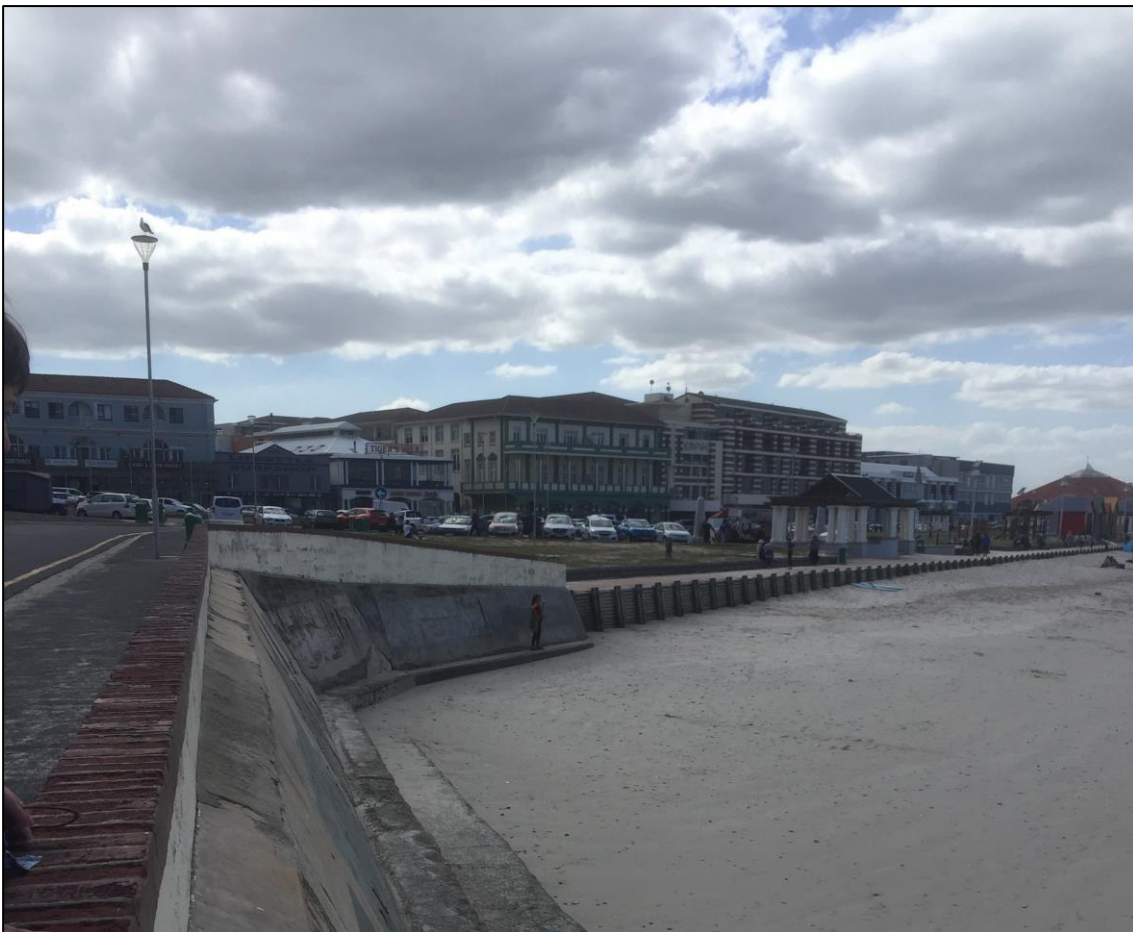
Plate 1: View north-east from the Point of the concrete walling and steps (foreground) and the timber revetment along the back of the beach that will be replaced (Photo: J Gribble).
