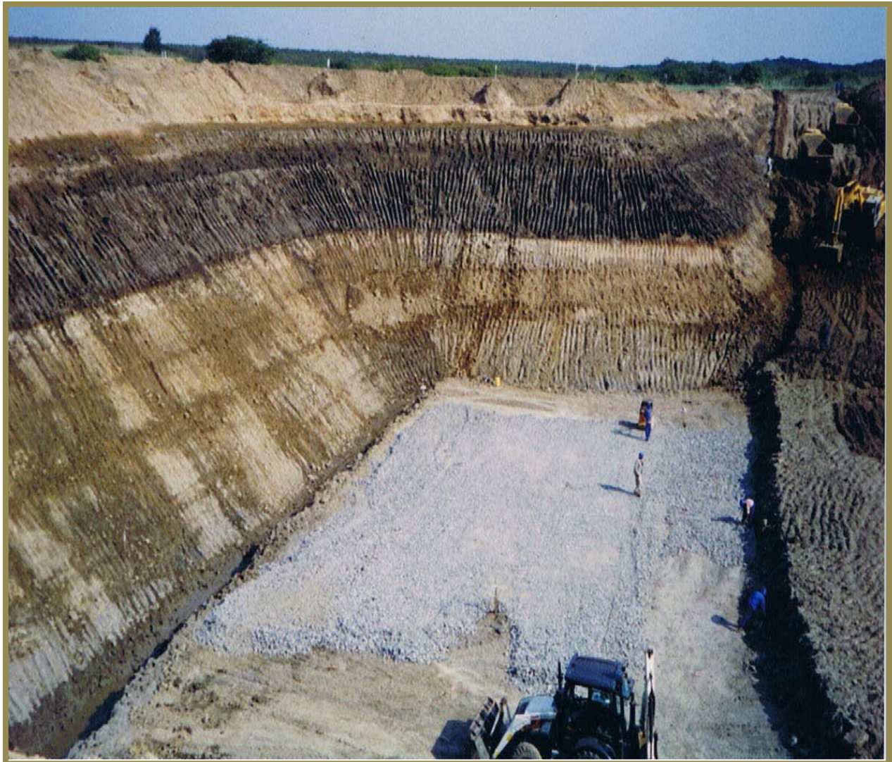
Figure 2 Excavations at Berth 306, Richards Bay Harbour. Exposure of Cretaceous horizons at 14m below m.s.l. 11
