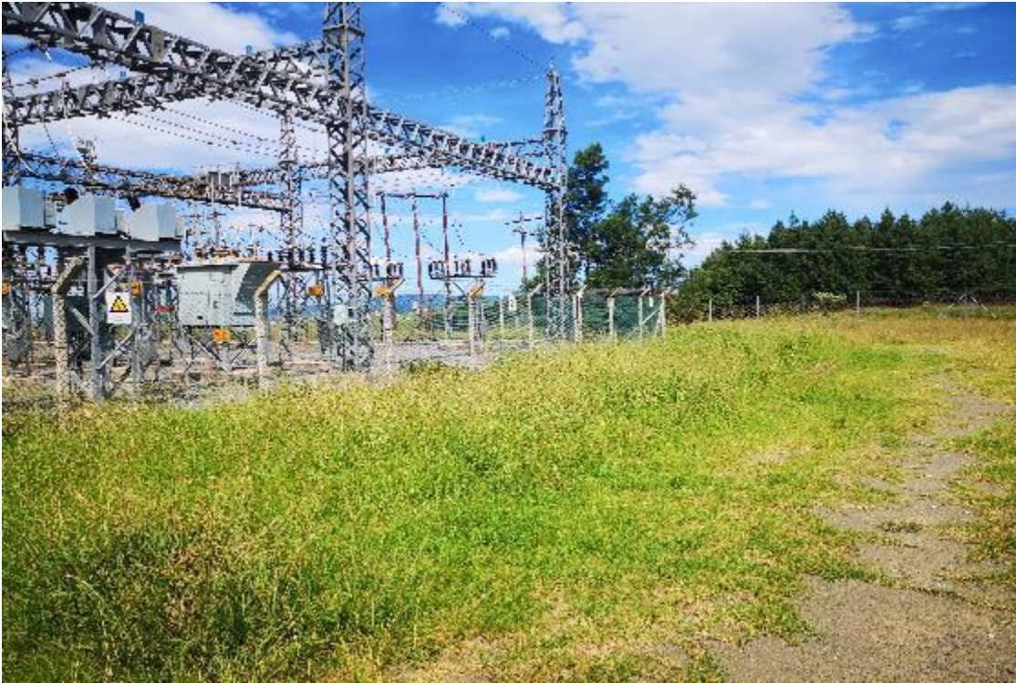
Figure 5: View of development area with substation
