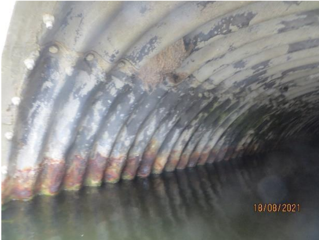
Figure 19: Corroded metal in cells
