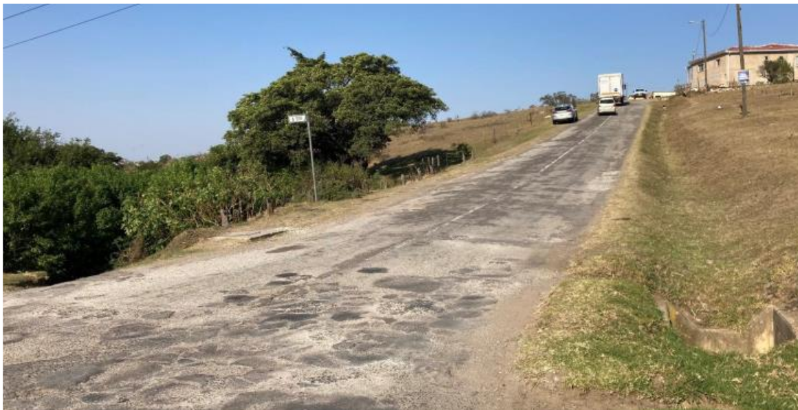
Figure 8: Typical view of road to be upgraded. Note the landscaped features consisting of cultivated grass and culverts.
