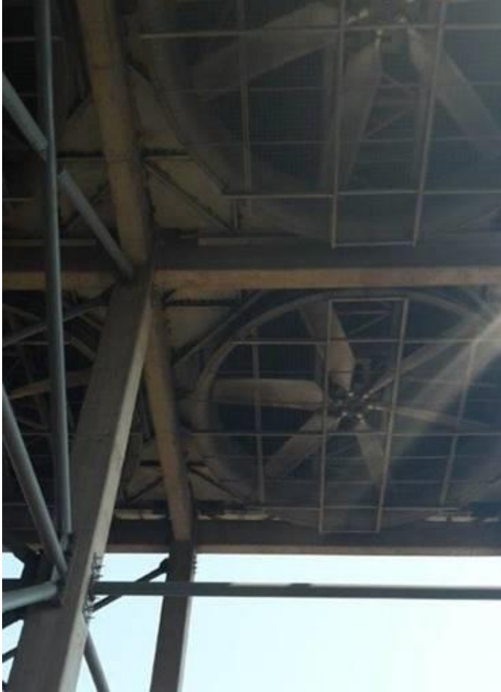
Figure 10: Air Cooled Condenser.
