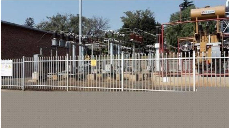
Figure 9: Tubatse's on-site Sub-station.
