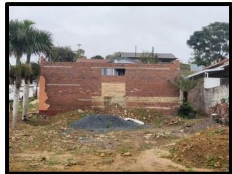
Figure 08: Ex. Dwelling – January 2022 roof structure and windows and doors stolen.
