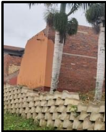
Figure 07: Ex. Dwelling – January 2022 Vandalized
