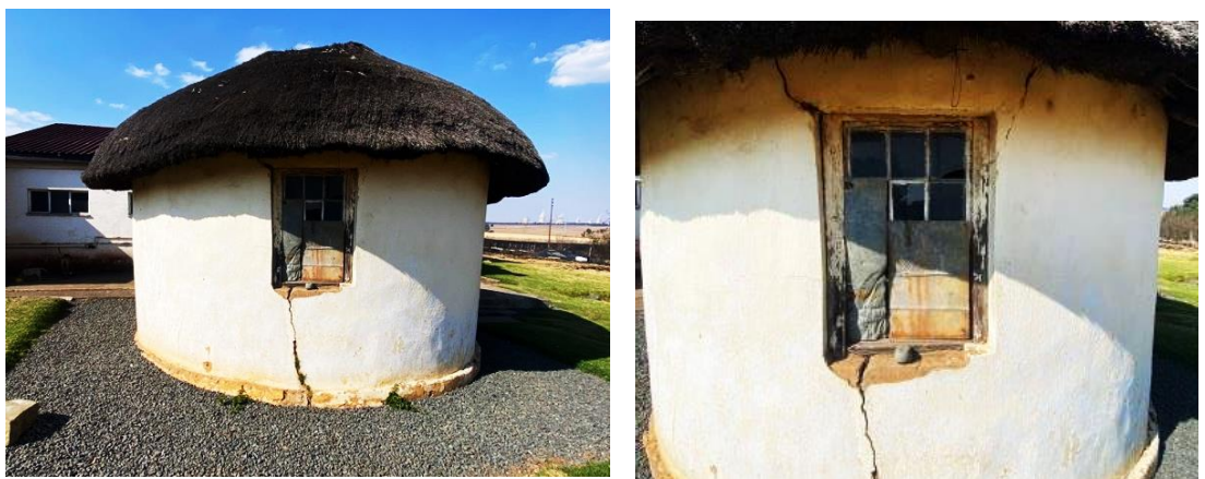
Figure 28. Detail of outside rondavel (west) showing wooden sash (six over six) detail as well as advanced state of pending collapse. (Photos S.U. Küsel 2023.)
