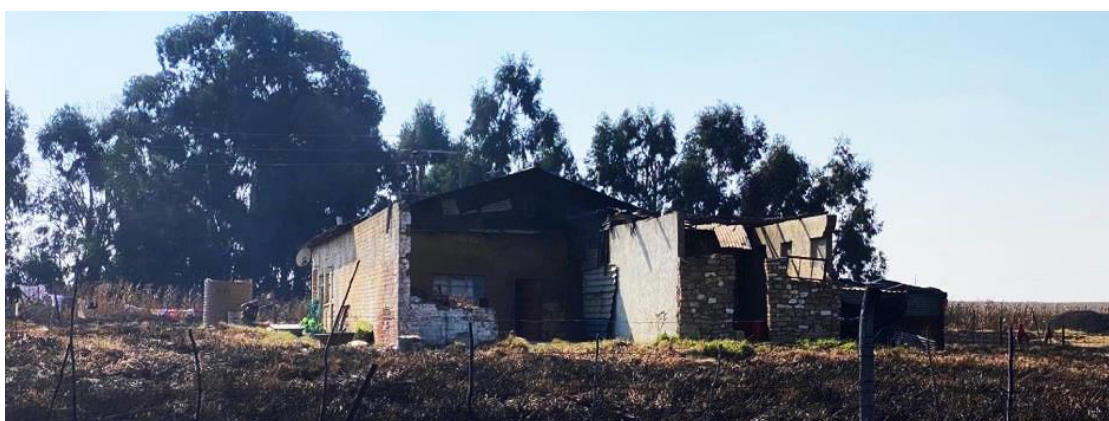
Figure 32. Former farm shed for machinery and storage that was partially demolished and then crudely altered and converted. It is now inhabited to being a “dwelling”. (Photo S.U. Küsel 2023.)
