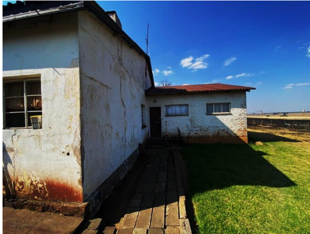
Figure 29. Back of farmstead from the south west showing steel windows modern door and both IBR and corrugated- iron roofing. It appears as if the foundation consists of a heavily mortared stone construction that is modern, rather than “old style” un-mortared stone construction. (Photo S.U. Küsel 2023.)
