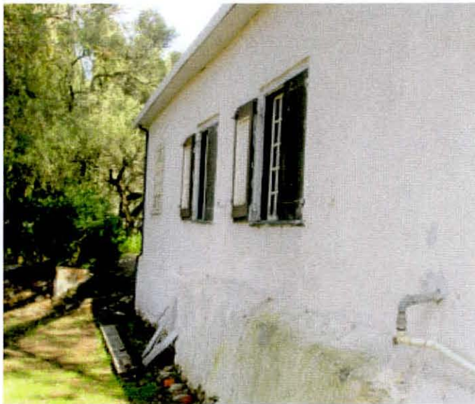
Figure B: Detail showing stone base of original cottage and damp penetration into plasterwork
