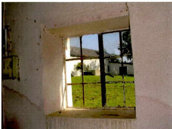
Figure D: Showing wall thickness, inserted metal-framed window and damp from interior of Mill House. Background building is the cellar.
