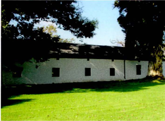
Figure A: Cellar from within the wharf showing high ground levels.
