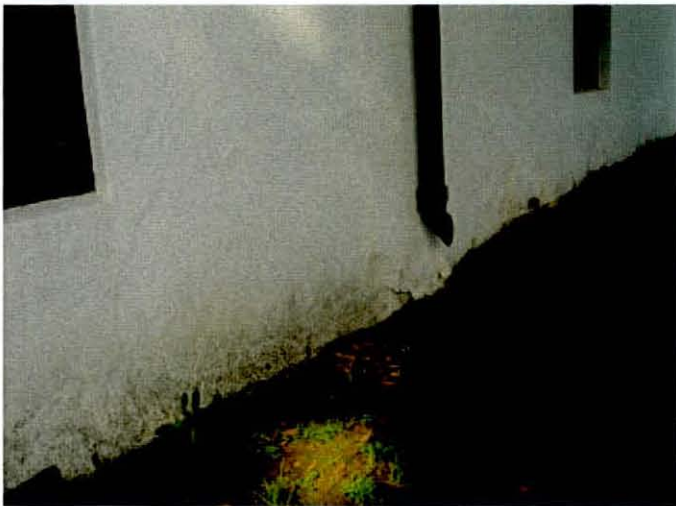
Figure B: Gutters with no dispersal system allowing damp penetration into old and porous walls. Some plaster cracking is also visible
