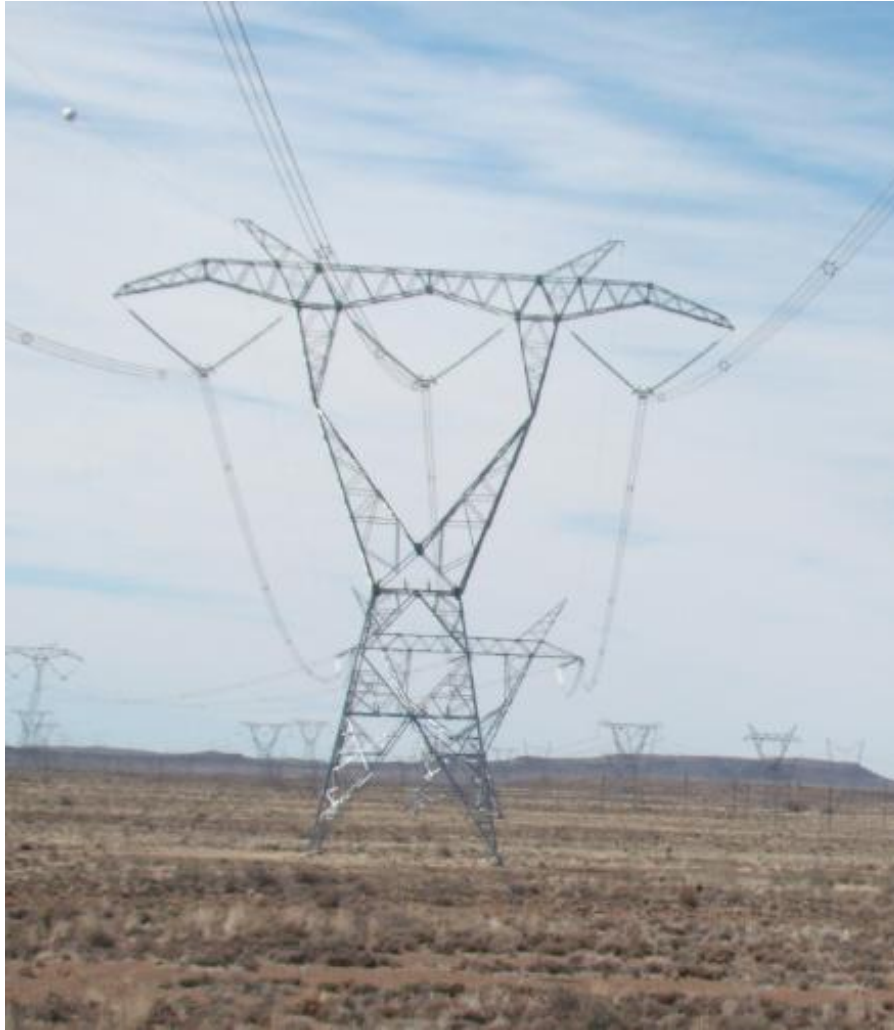
Plate 10: Self Supporting suspense tower (H. Mlotshwa, 2013)
