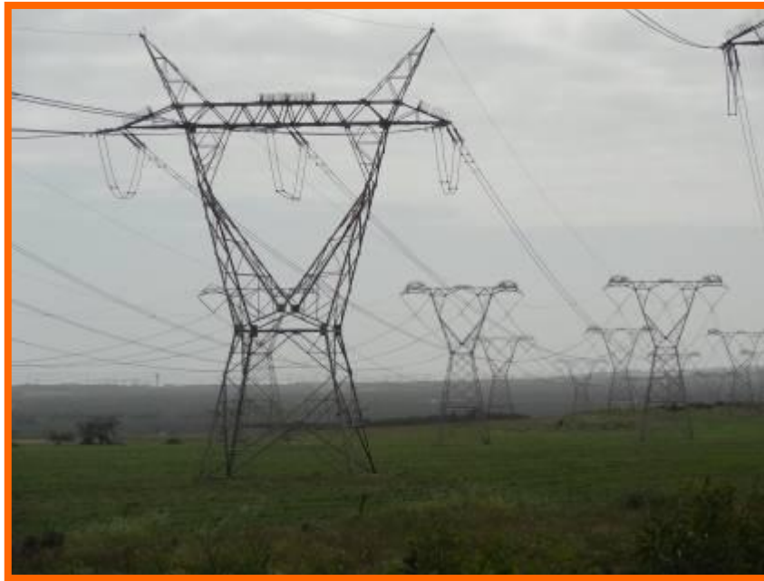
Plate 1: Self-supporting strain tower(Photography: H.Mlotshwa 2013)
