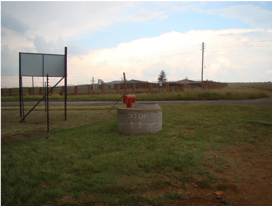
Fig. 12: The point where the pipeline will connect with the tarred road from the dirt road (west), cross it, and change direction (from here it will turn north to follow along the tarred road, fig. 10 & 11).
