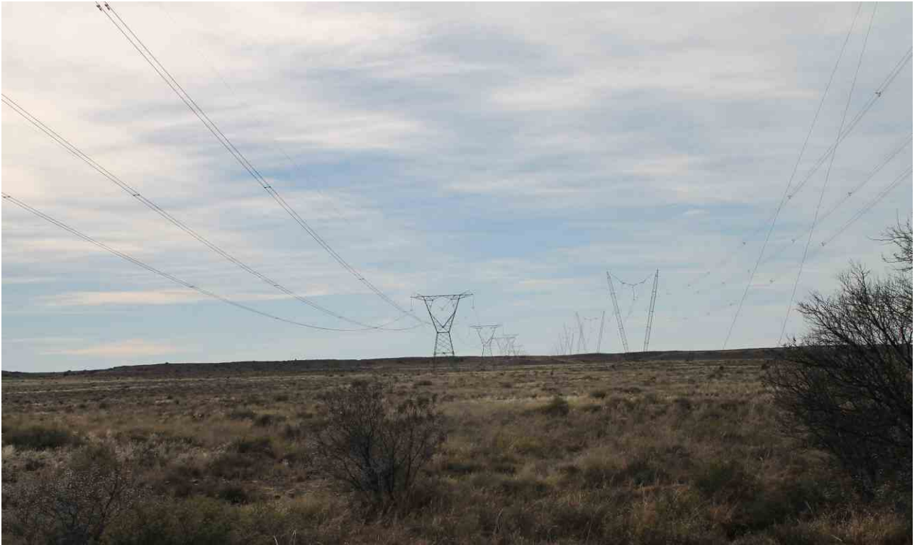
Figure 3 An example to two kinds of 400 kV lines and towers. Left: conventional self-supporting towers. Right: guyed "V" towers or compact crossrope towers. Guyed "V" towers have a very small ground surface footprint and are more easily absorbed against a skyline.
