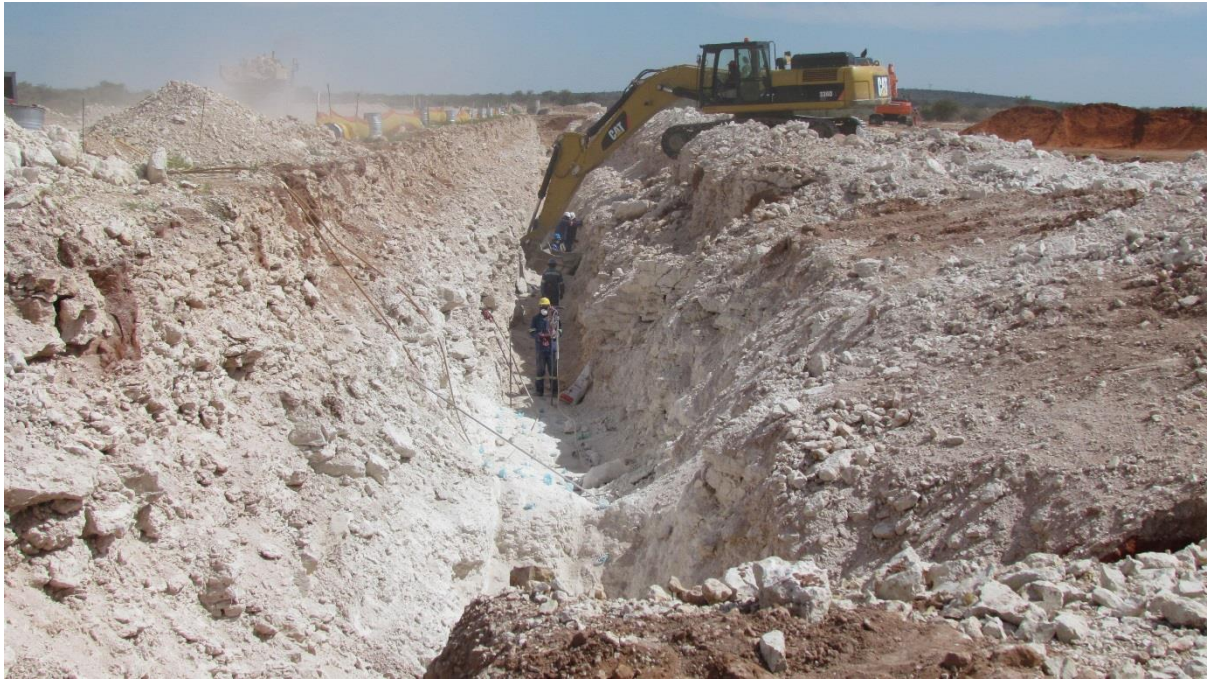
Deep trenching at point GPS 290, indicating at least a few metres thickness of calcrete.
