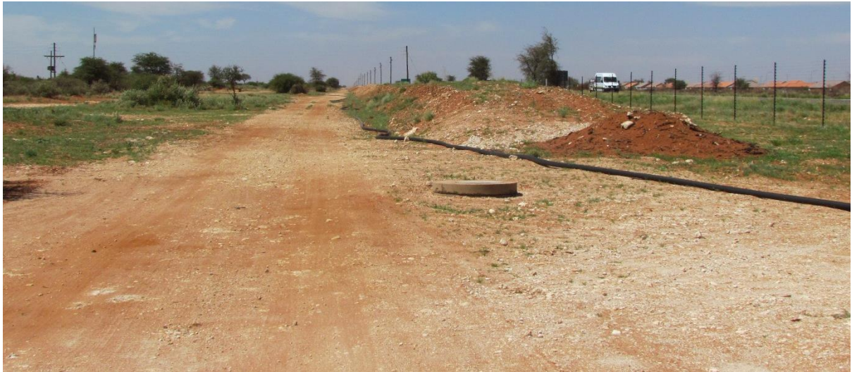
Pipeline route (above and below): no archaeological deposits were in evidence at any point.
