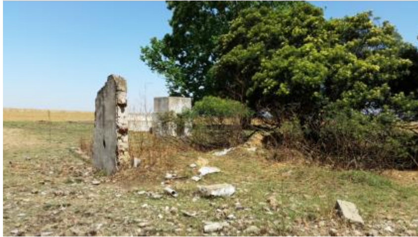
Figure 3-4: Ruined structure (S.34-007)
