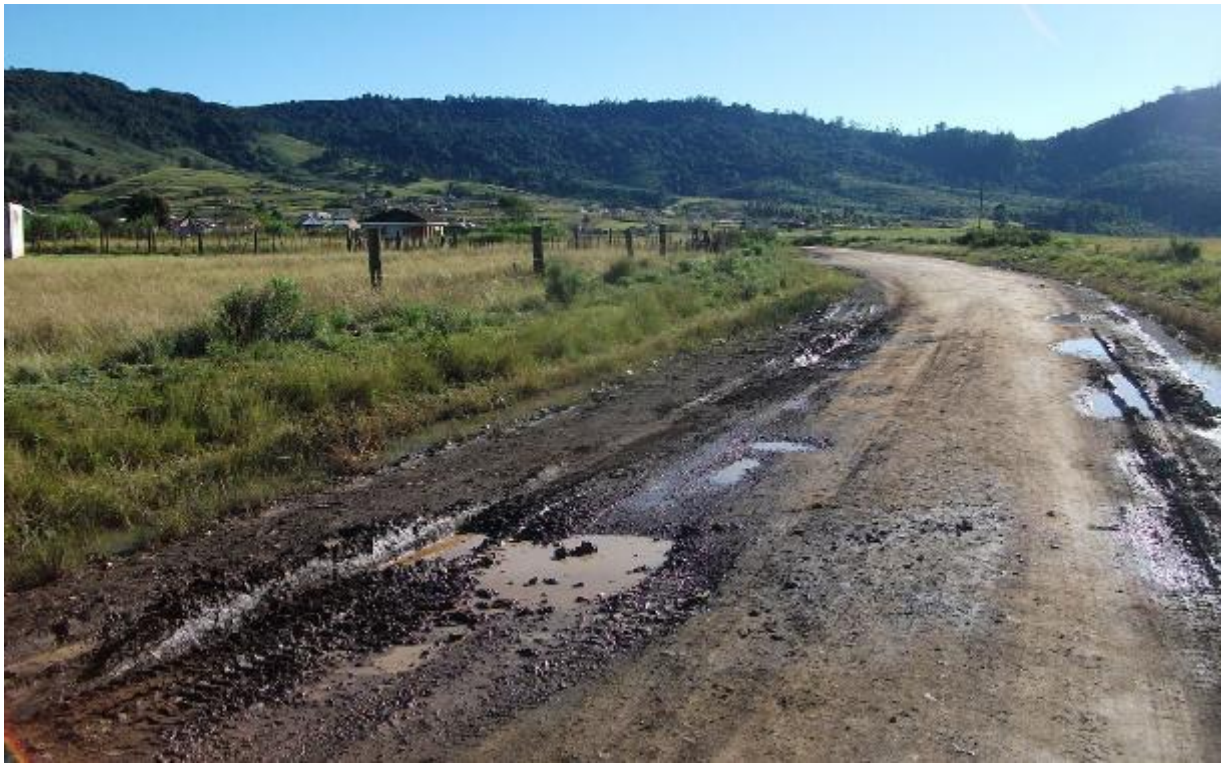
Figure 5: View of condition of Baleni Road looking northwards
