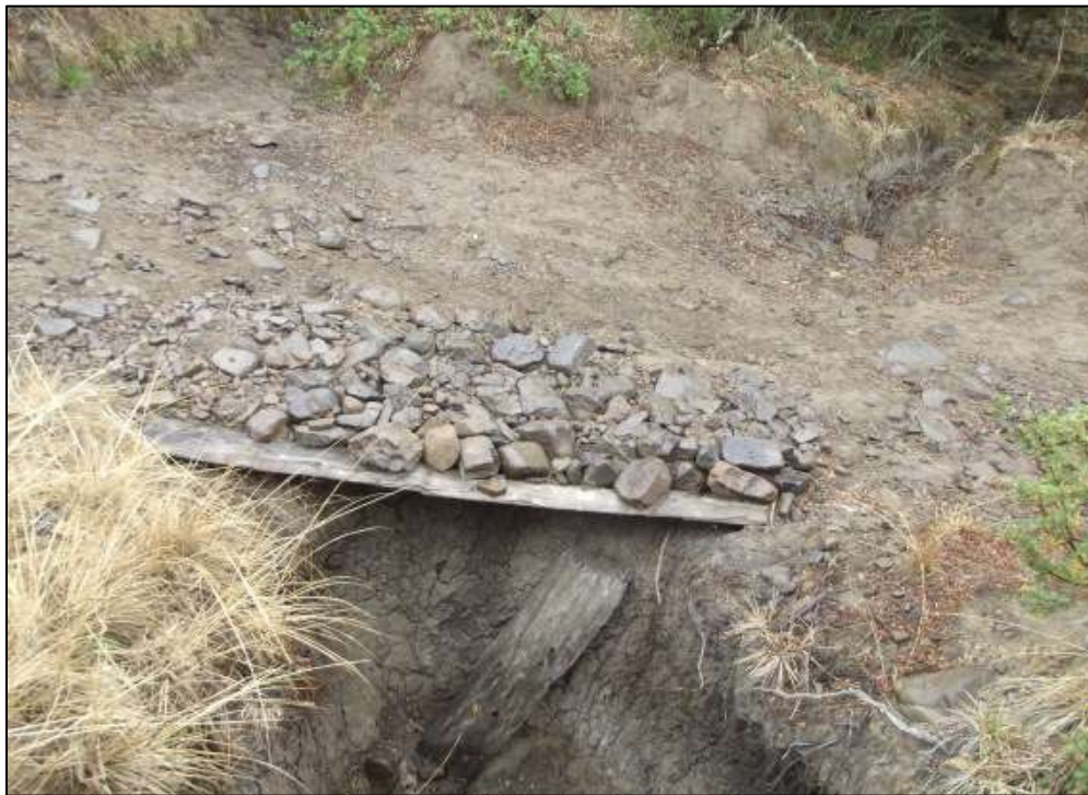
Fig. 17. Site WB 8. An historic bridge or crossover. Note the railway sleeper at the bottom, it was probably part of the original structure.
