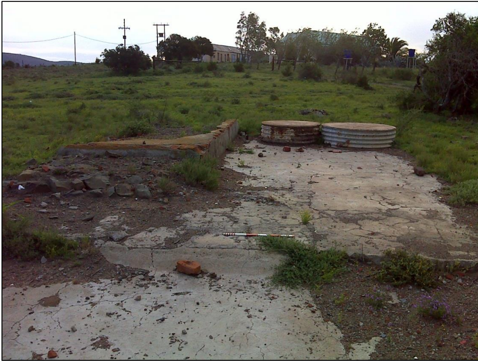
Figure 23. View of the foundation of the remains of a building (SK BE1)
