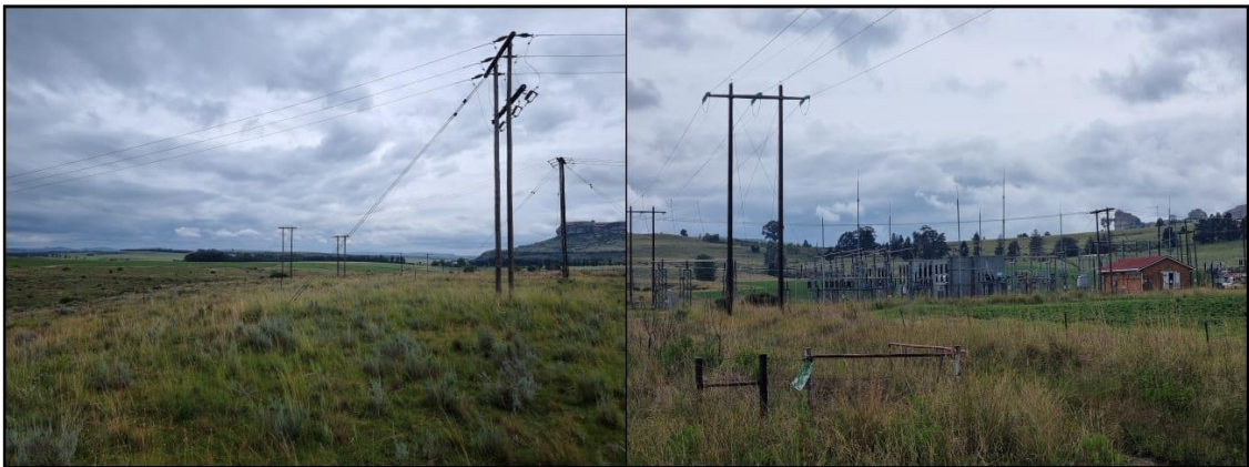
Figure 5-6: View of ESKOM powerlines and the Node Substation (right) in the project area.
