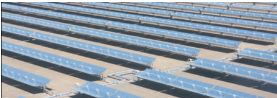
Figure 4. Reflective solar plants (parabolic troughs)
