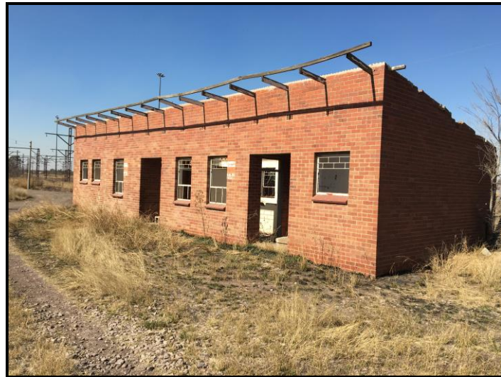
Figure 23. Ruin of bathrooms.
